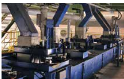
Weighing and dosing units (4)
