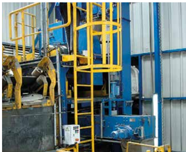
Sampling system for copper concentrate
